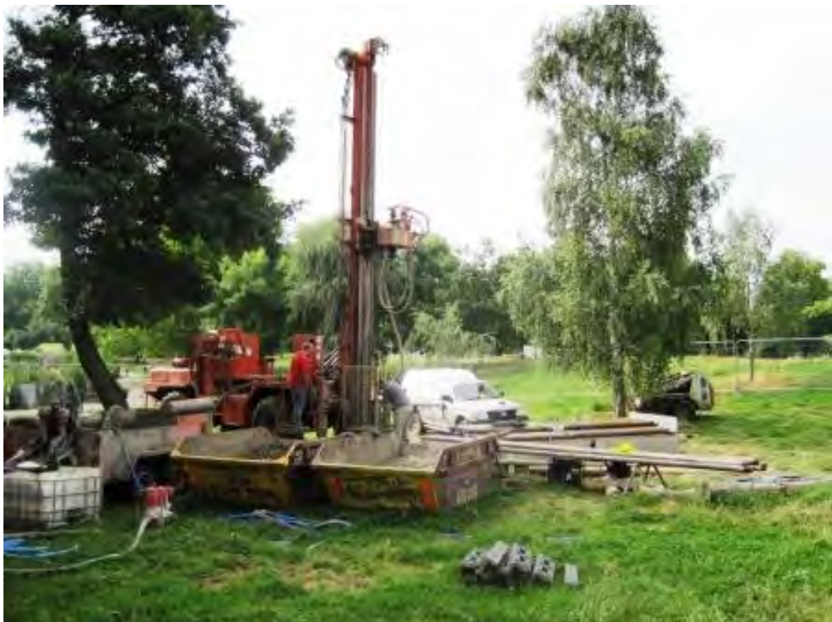
Figure 69. Drilling a new groundwater borehole next to Mount Pond on Clapham Common to reduce dependency on a mains water supply (London Borough of Lambeth)
