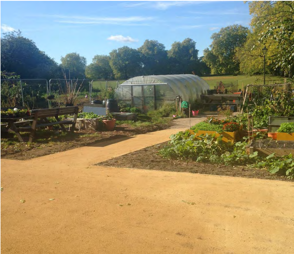
Figure 47. New compacted gravel paths within the community garden on Clapham Common to provide safe public access (Clapham Common Bandstand Beds)
